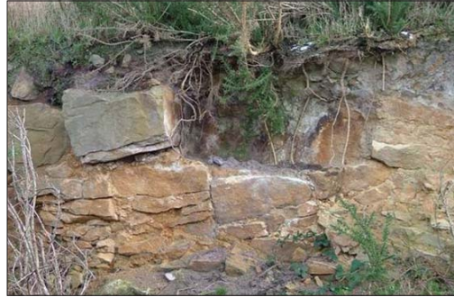
▲ Example of unstable rock faces at Woodside Quarry
